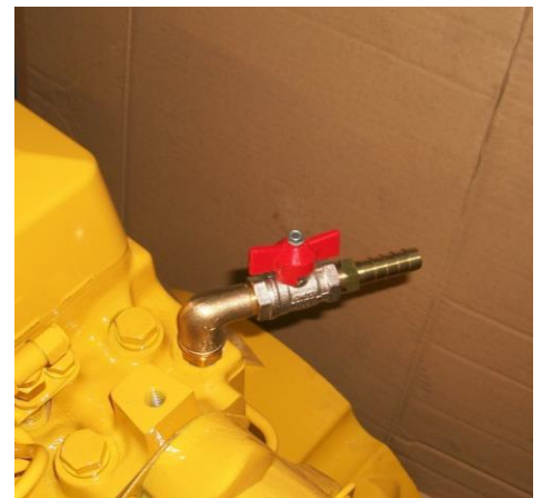
Calorifier Outlet (located on rear of engine)
